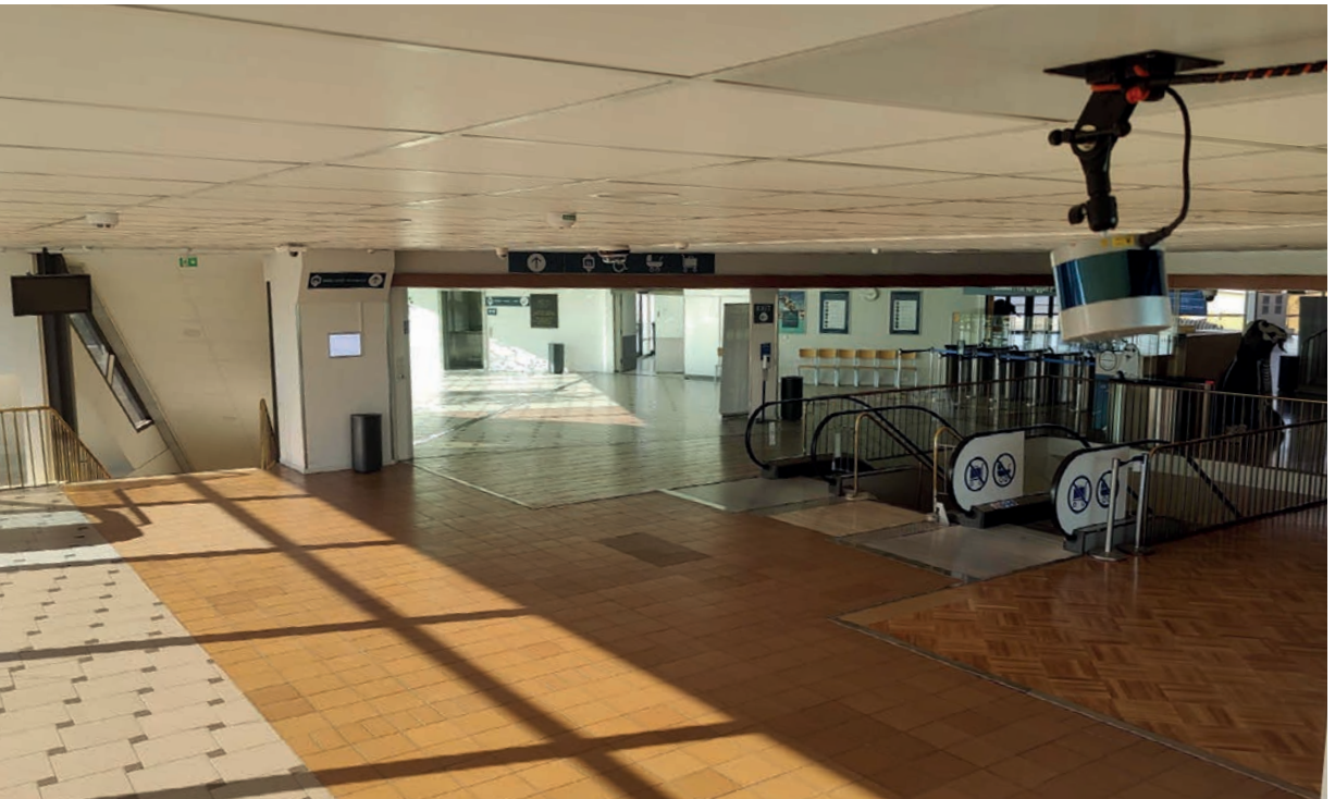
Figure 1. Installation of the lidar sensor and indoor base station (top of the pole, on the right).
